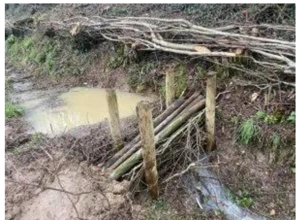
Figure 19 Example of a functioning Leaky dam holding back water (image credit Vicky Whitworth
